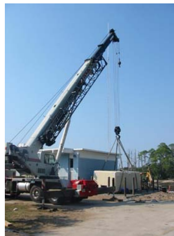
New gas tank
